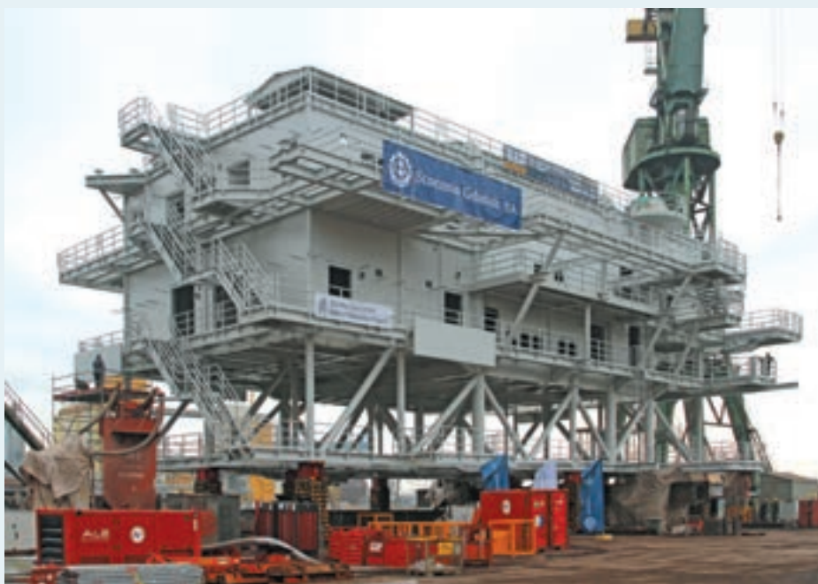
The "trafo-platform" from the Gdansk Shipyard has been among the largest one structures of this kind built in Poland so far.
