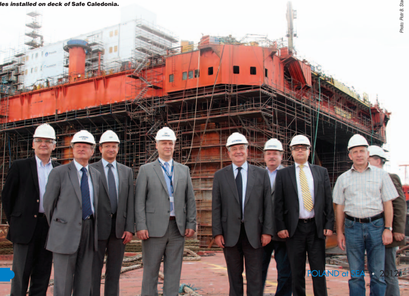
Representatives of the Supervisory Board, the Board of Directors and the shipyard's management. In the background - new accommodation modules installed on deck of Safe Caledonia.
